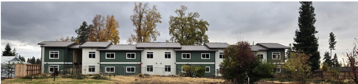
Photo of construction progress (back of building as seen from Rosemary Court)
