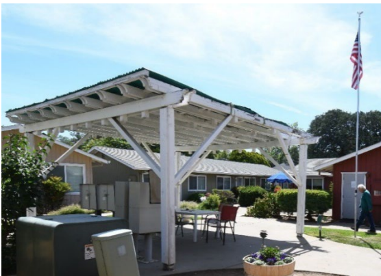
Pergola slated for replacement
