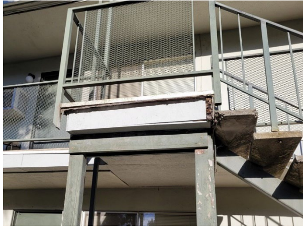
Upper level stair landing slated for repair
