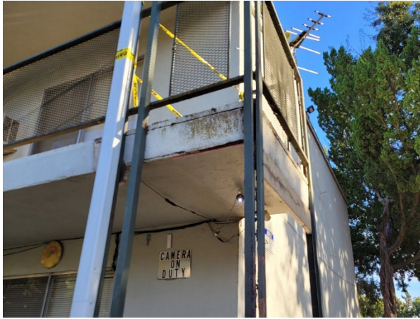
Upper level walkway slated for repair
