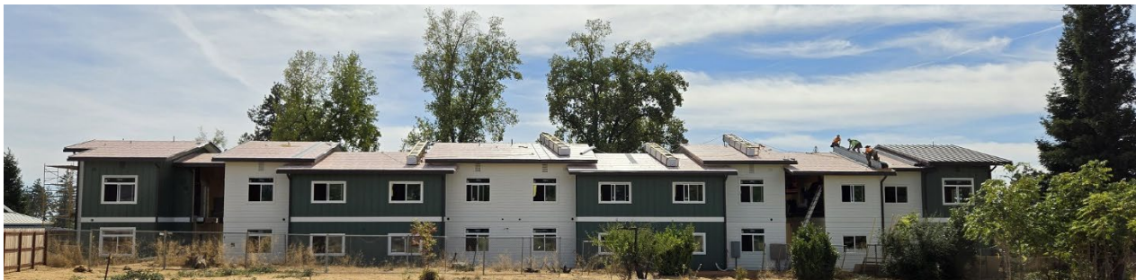
Photo of construction progress (back of building as seen from Rosemary Court)
