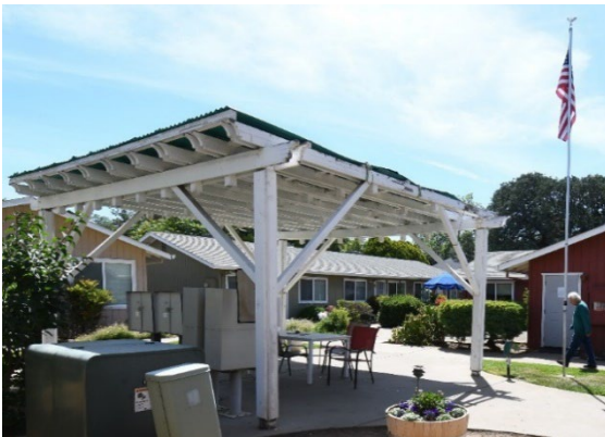
Pergola slated for replacement
