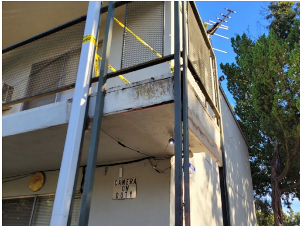
Upper level walkway slated for repair
