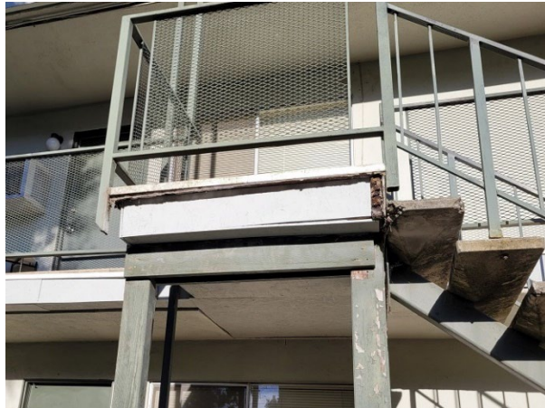
Upper level stair landing slated for repair
