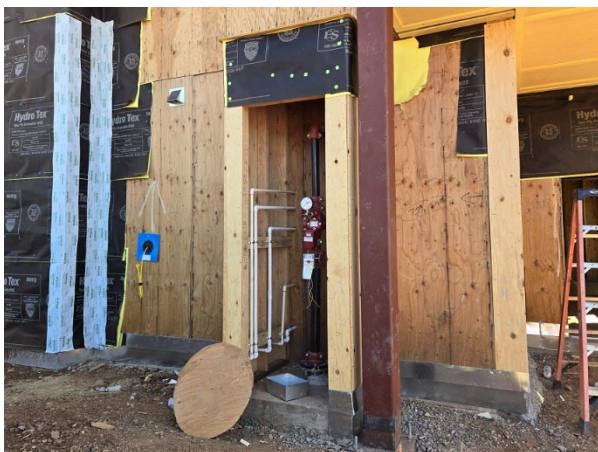
Fire Suppression Riser Room
