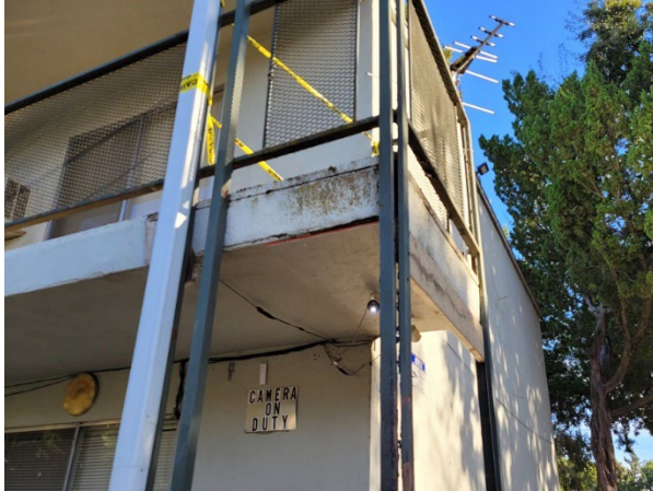
Upper level walkway slated for repair
