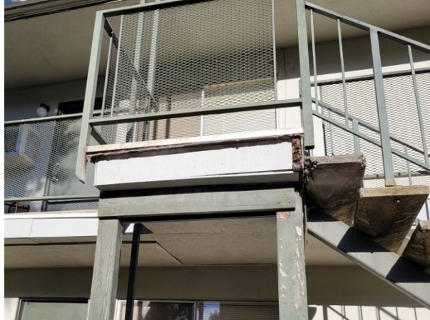
Upper level stair landing slated for repair
