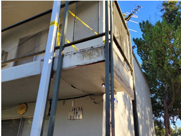
Upper level walkway slated for repair
