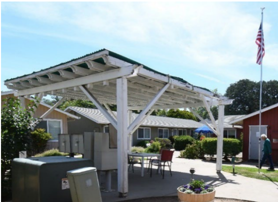
Pergola slated for replacement
