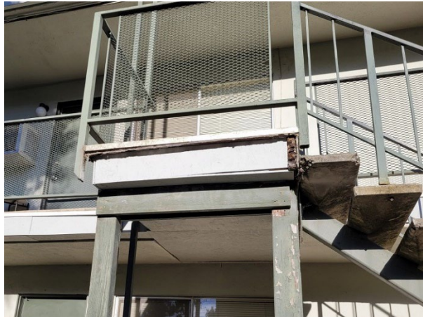
Upper level stair landing slated for repair
