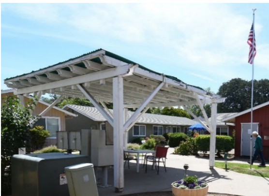
Pergola slated for replacement
