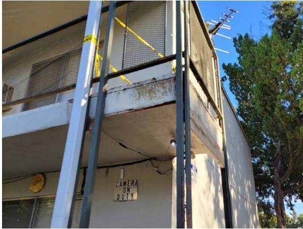
Upper level walkway slated for repair
