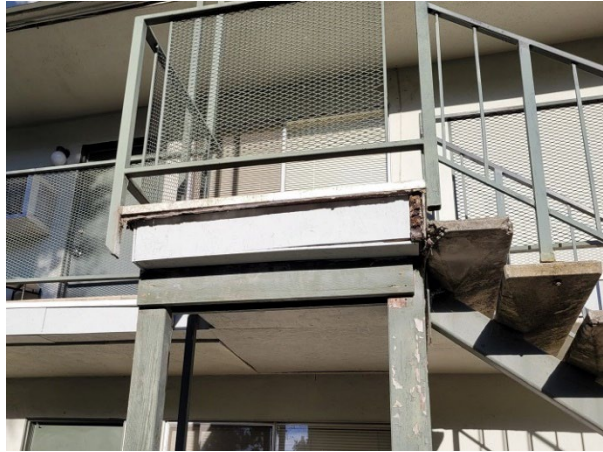
Upper level stair landing slated for repair
