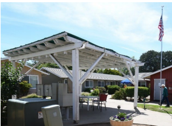
Pergola slated for replacement
