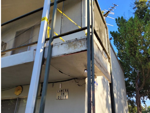
Upper level walkway slated for repair
