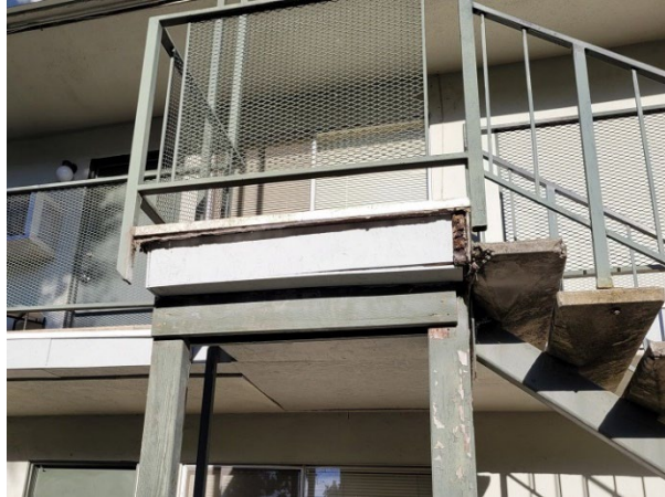
Upper level stair landing slated for repair
